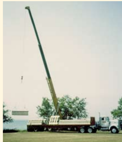
Shore-based installation is the most cost-effective method
